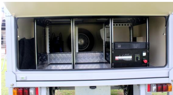
SAT-2000 a integrated with manual positioner, UPS and power distribution, air conditioner and equipment racks, on HMT-2000 semitrailer.
