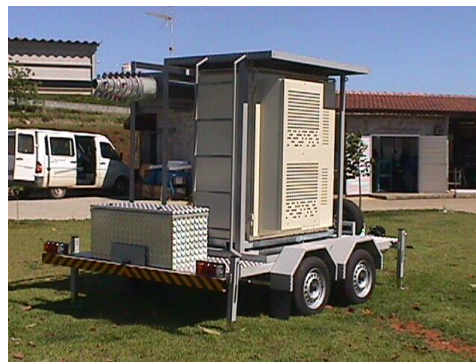
With 18.3m mast and Motorola 4812LT BTS
