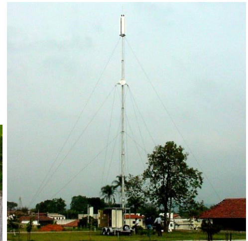
With 18.3m mast and Motorola 4812LT BTS, guyed mast
