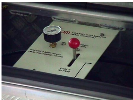
Control panel detail with the system installed
